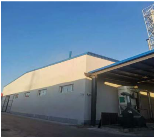
车间燃气锅炉废气烟囱
